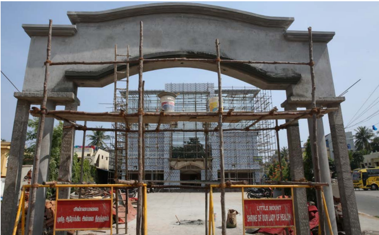
Le chantier de rénovation de « St Thomas Community Hall ». Work during renovation of St Thomas Community Hall, Little Mount, Chennai, 2020
